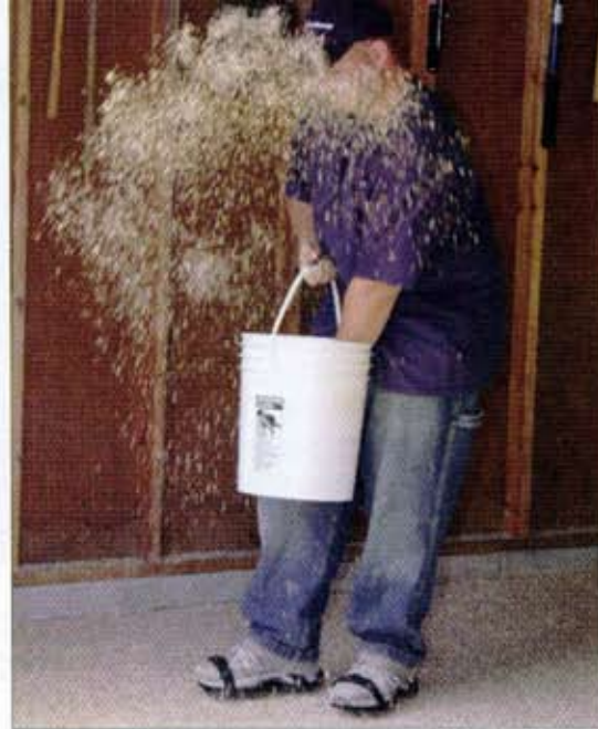
Wearing cleats, a worker walks immediately into the polyaspartic polyurea bedcoat to broadcast the 1/4-inch vinyl chips. Tossing the chips upward delivers a consistent finish with a wide chip-spread.
